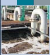
INDUSTRIAL WATER TREATMENT
